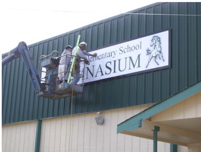
Custodian Brian Cooney (L) assists Rich Quigley (R) of DCI Builders install the new sign on the school gym.
